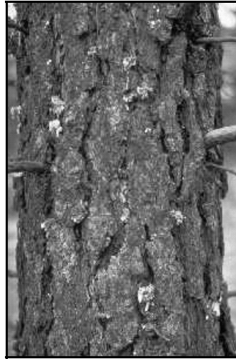
MPB "pitch tubes" Photo Courtesy of Fire Ready
